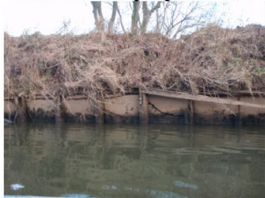
Downstream length: cracked wall
