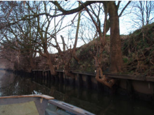
Downstream length: tree damage
