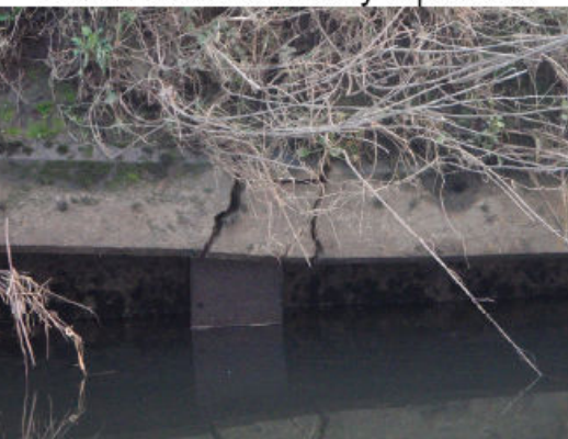
Upstream length: failed repair, replacement required
