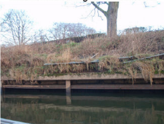
Upstream length: hole in bank covered with steel mesh fence
