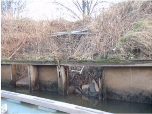
Downstream length: hole in wall & bank
